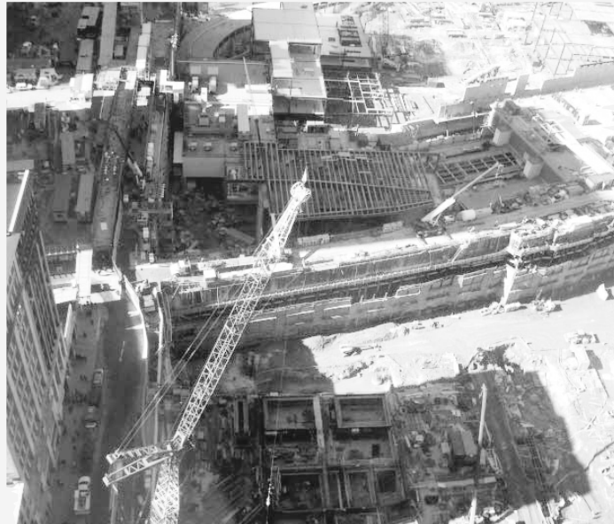
Foundation of Tower 4 (bottom of picture) and South Tower Memorial (top) at Southeast corner of site.
