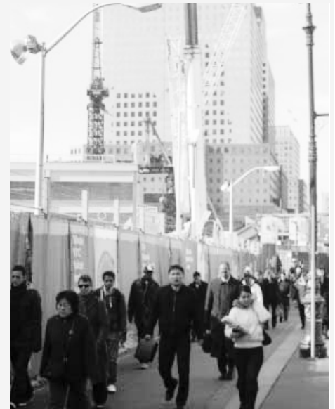
NJ commuters are diverted around site to temporary Path train station at north end.
